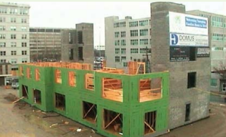
Construction on the Family House began to take shape at 4th & Callowhill this March.
